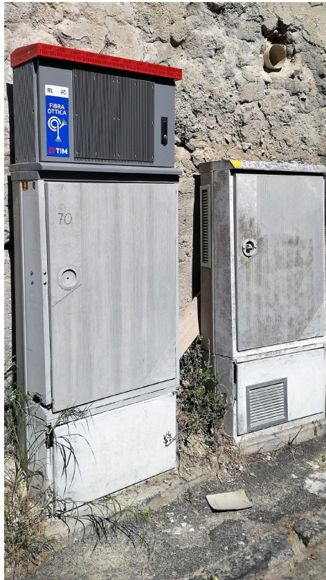
Figures 17–18: An abandoned cabinet of the Socrate project and a re-used one, in Naples.
