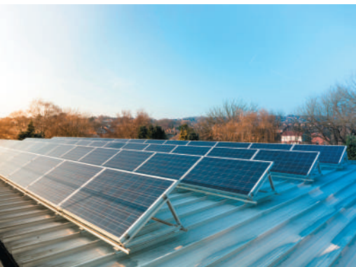
Figure 32.18 These rooftop solar panels are tilted to be face-on to the sun—that is, face-on to the Poynting vector of electromagnetic waves from the sun, so that the panels can absorb the maximum amount of wave energy.
