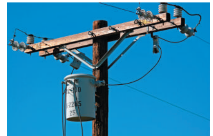
Figure 31.22 The cylindrical can near the top of this power pole is a step-down transformer. It converts the high-voltage ac in the power lines to low-voltage (120 V) ac, which is then distributed to the surrounding homes and businesses.
